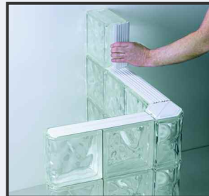
4 » Using both the horizontal and vertical spacers, your next row of glass block is ready for installation.
